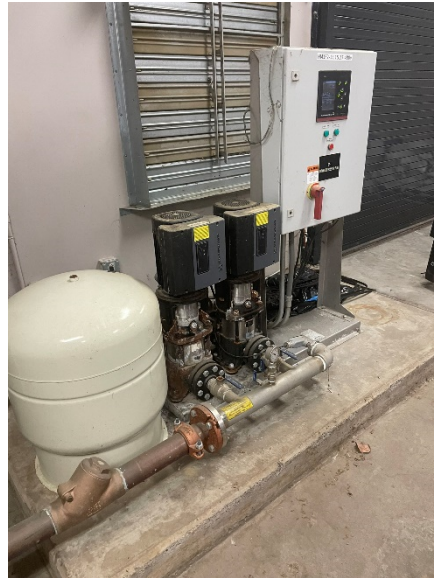
Figure 14: Rainwater Recovery System
