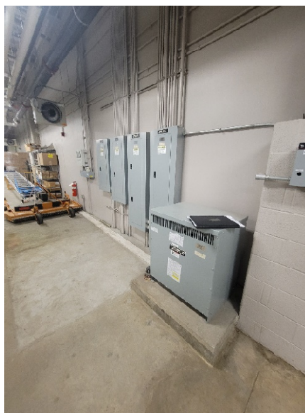
Figure 12: Panels and Transformer
