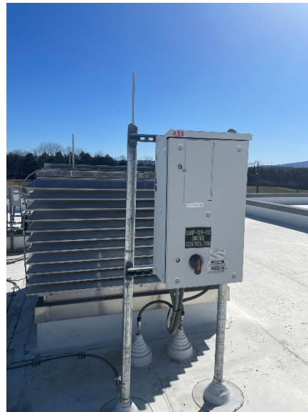
Figure 6: Smoke Control System Fan
