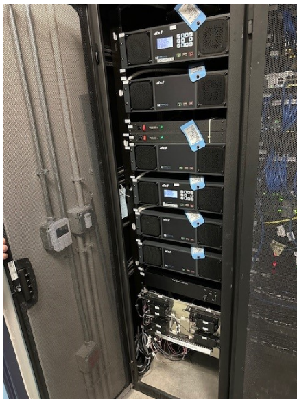
Figure 19: Security System Head-End
