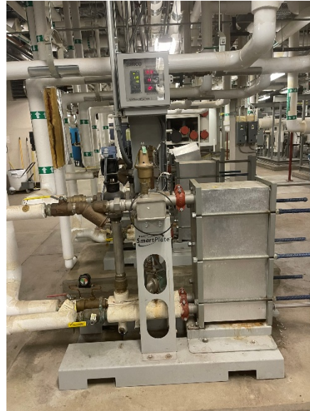
Figure 16: Domestic Water Heater Exchanger
