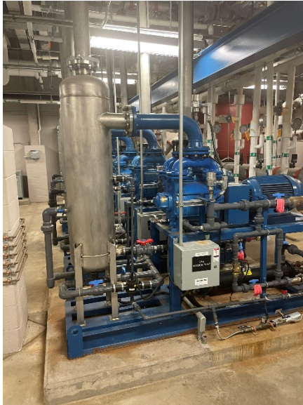
Figure 15: Vacuum System Pumps
