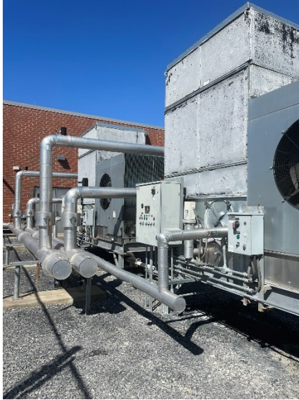
Figure 1: Closed Circuit Cooling Towers
