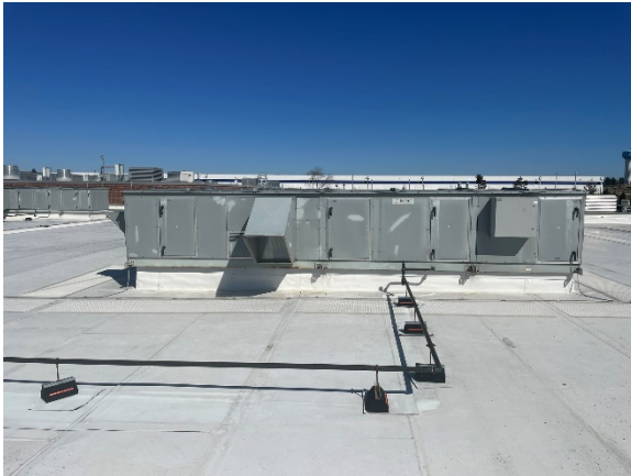
Figure 3: Rooftop Air Handling Unit
