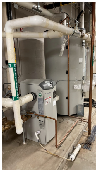
Figure 17: Domestic Water Heaters
