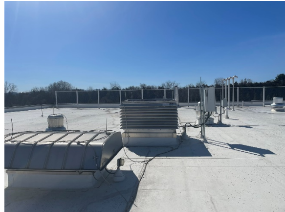
Figure 4: Exhaust and Filtered Supply Fans
