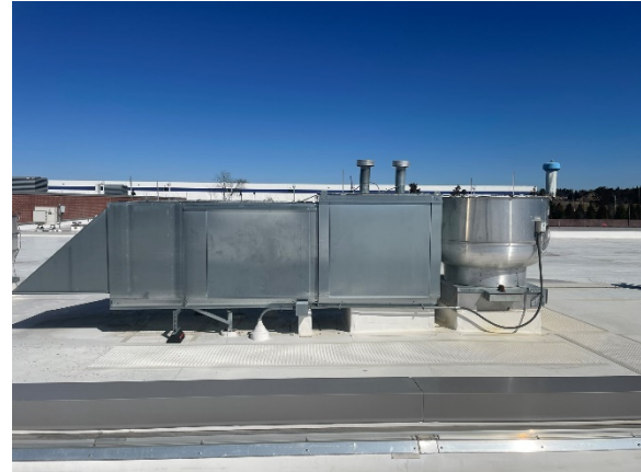
Figure 2: Makeup Air Unit and Exhaust Fan
